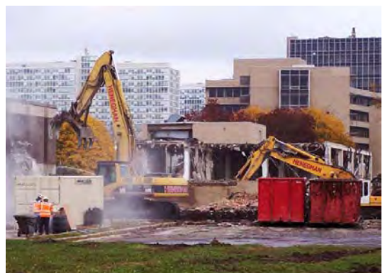
East elevation of the Friend Convalescent Home, MRH campus, and below, demolition in October 2009.
