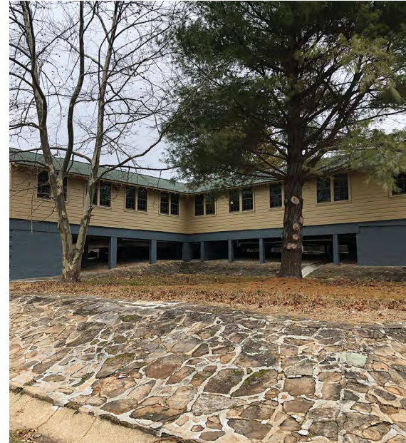
The completed rear elevation of Building 2101 at Fort Leonard Wood, MO and restored retaining wall features stonework completed with German prisoners of war labor.
