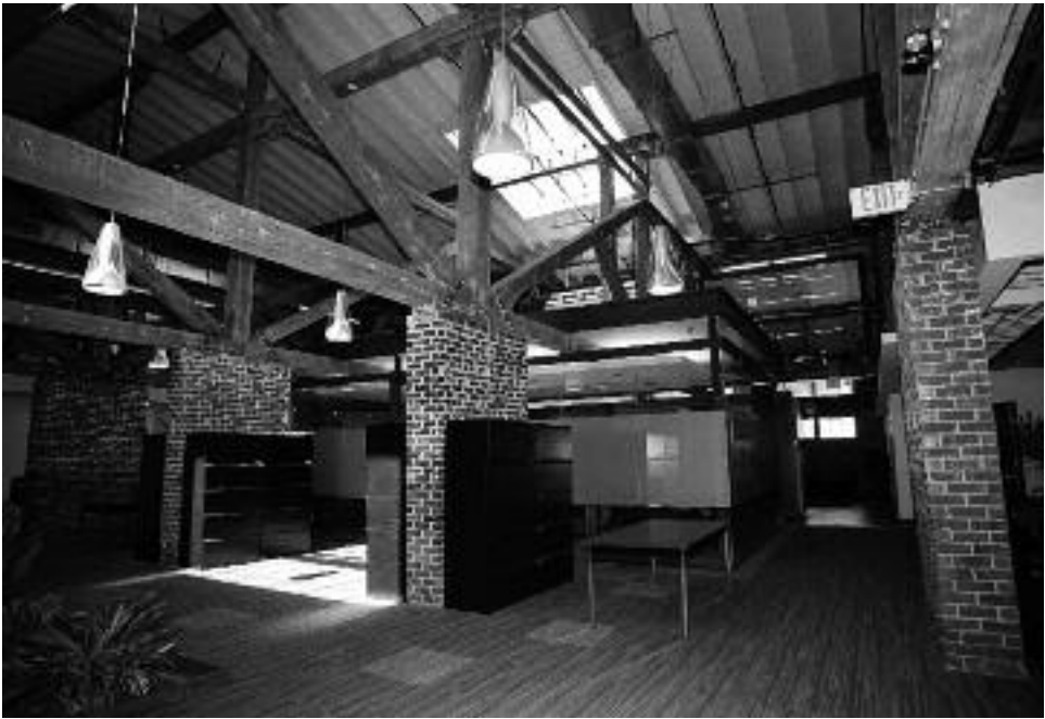
The conversion of this former manufacturing building in Richmond, Va., into law offices makes striking use of the 1905 structure's original, character-defining features—notably the heavy-timber trusses. Photos courtesy of the National Park Service.
